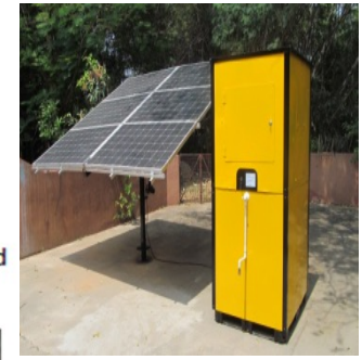
Water Kiosk & Solar Panel
