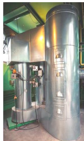
ATON MOS system for neutralization of exhaust gases from sintering line
